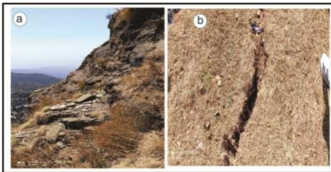
Figure 4: (a) highly shattered and jointed condition of rock mass exposed at crest of Naini Hill (b) tension cracks on the crown of Naini peak
