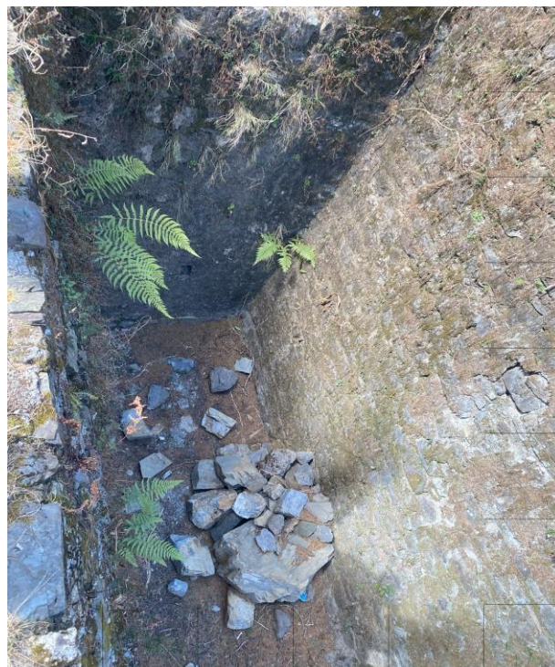
Figure ... The slided rock pieces obstructed by the retaining wall
