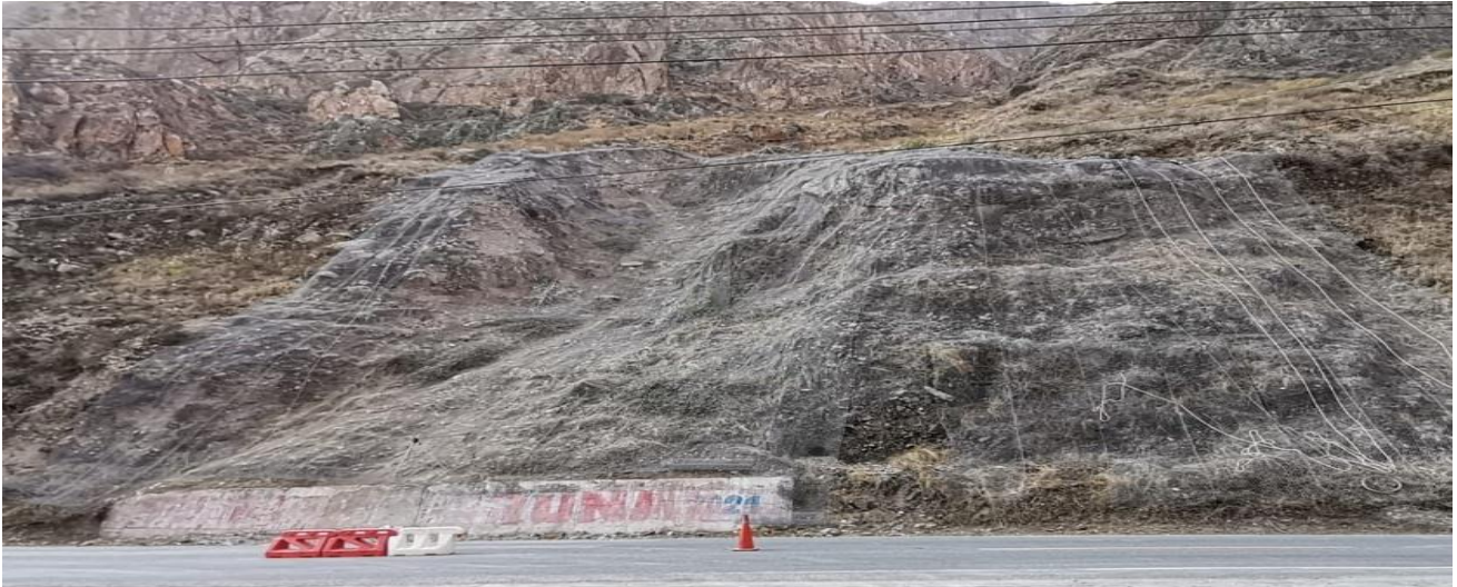
Figure 10: Wire Meshing Protection Nets
