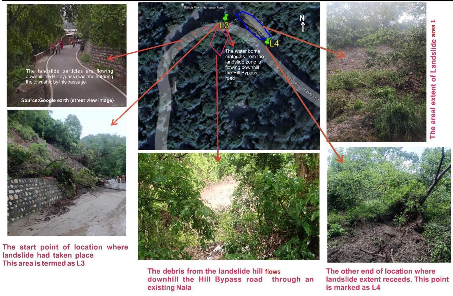
Fig. 4: Google Earth image showing the location of the first landslide, situated along the Hill Bypass road, points L3 and L4 mark the start and end point of the landslide stretch. It is also observed that landslide materials accompanied by water are flowing downhill in S (continuing straight by the road into an existing Nala) and SW (down the road into the township) direction. Each point marked in the Google Earth image is explained with respect to field photographs.
