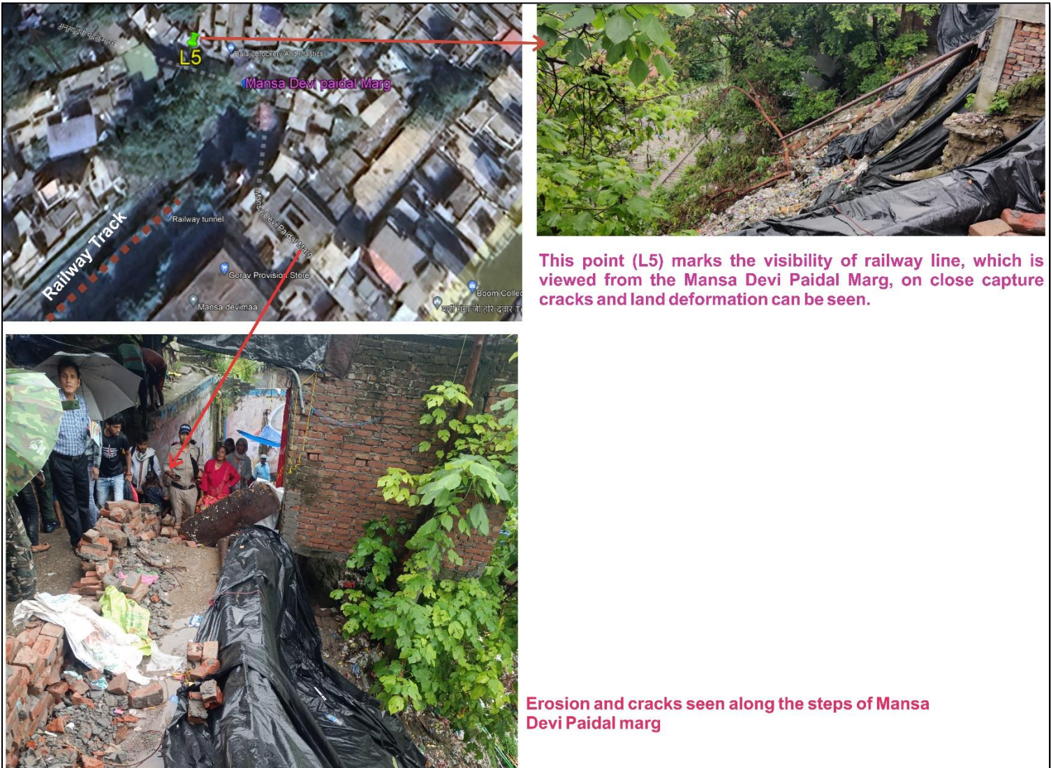
Fig 6: Google Earth image shows location L5 situated along the railway track, which is visible from the Mansa Devi Paidal Marg. It is observed that around L5, there is an accumulation of moist rock and mud fragments which is apparently adding an erosion effect to the surrounding. Likewise, the steps of Mansa Devi Paidal marg are also eroded and cracks appear in places. Each point marked in the Google image is explained with respect to the field photograph.
