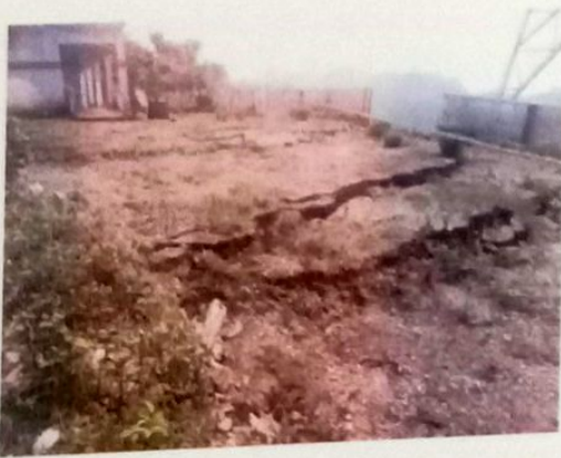
Crack on Ground of Government School
