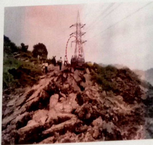
Damaged Transmission line Tower
