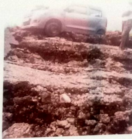
Ground Settlement along the longitudinal cracks
